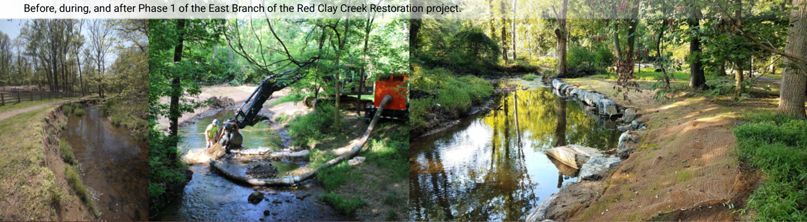
Before, during, and after Phase 1 of the East Branch of the Red Clay Creek Restoration project.
