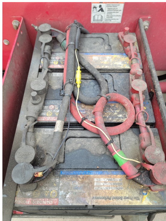
Battery needs to be cleaned
