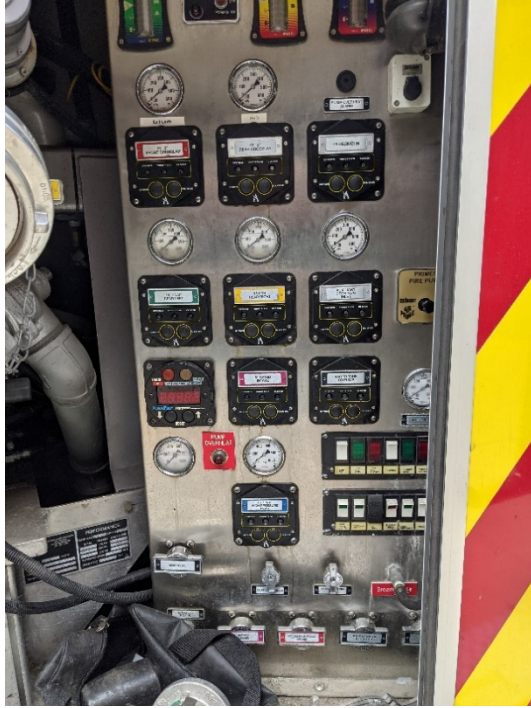
Electronic pump panel was costly and not needed.
