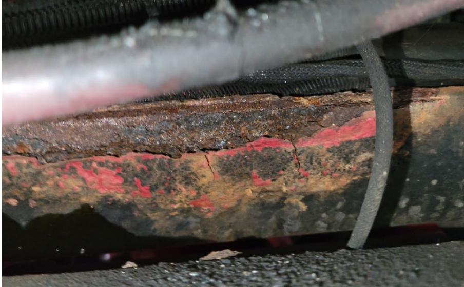
The frame rails are rusting and delaminating on Engine 251
