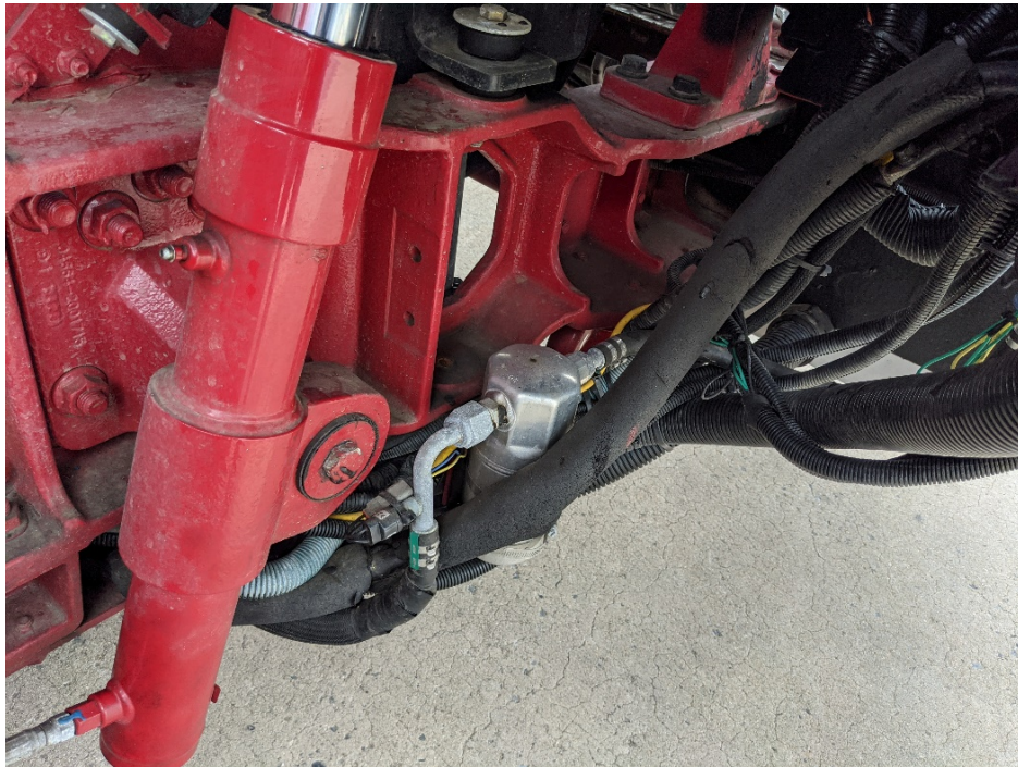
Repair the chaffing on the hose and the cab.
