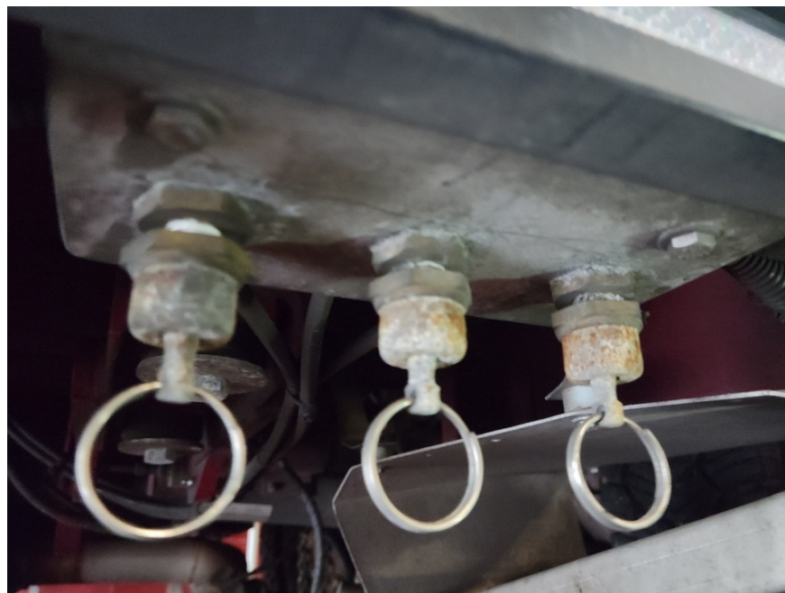
Underside corrosion needs to be mitigated.
