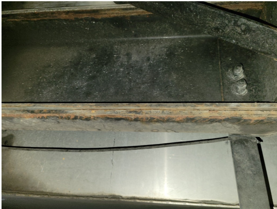
Rust, corrosion, and dirt accumulating on the frame rails.
